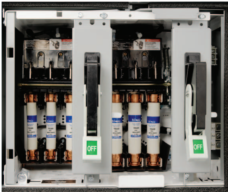
Example of Dual Feeder Disconnect Switch (DFDS)
