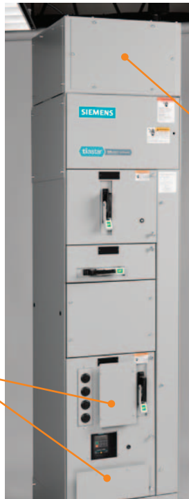
Figure 2. Closed Door View - Arc Resistant MCC
